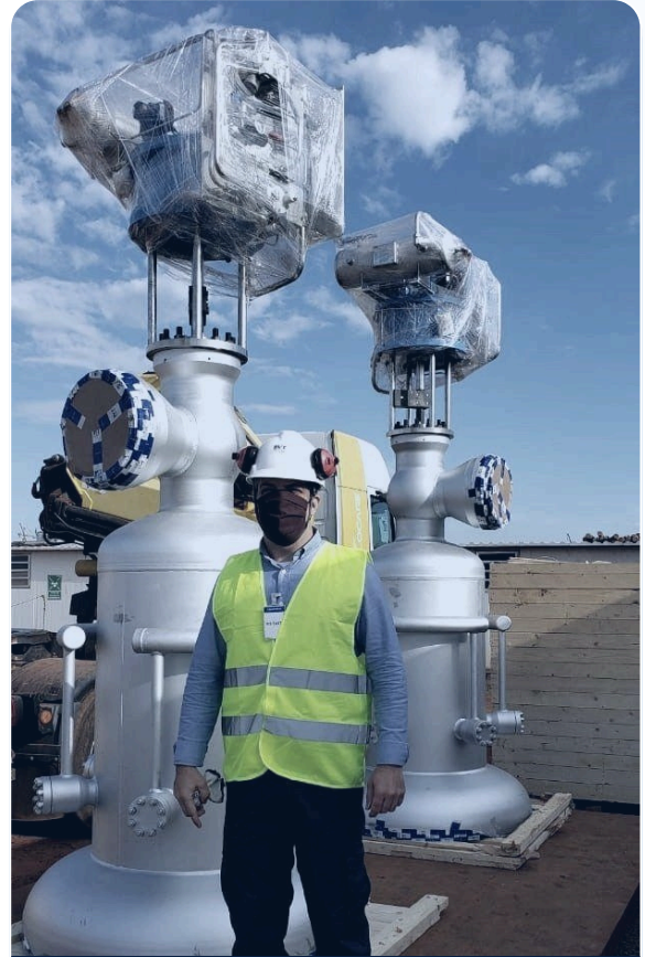
Bypass valve installed on site
