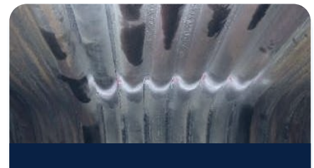
Superheater tubes in waterwall boilers
