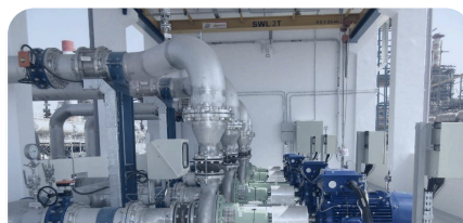
Booster pumps (3 working + 1 standby)
