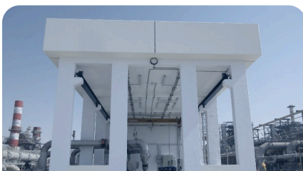
Booster pump station
