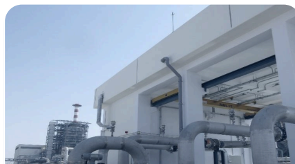
Pump station exterior
