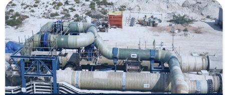
Pipework and pipe racks
